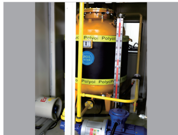
聚醚+环戊烷混合后储存系统 Polyether + cyclopentane mixed storage system
