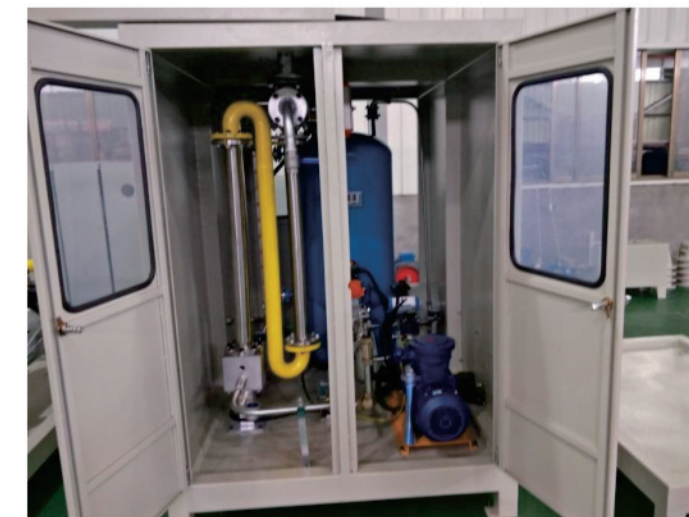
静态混合室 Static mixing room
